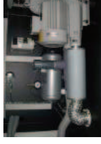
Ring blower inside the purge compartment
